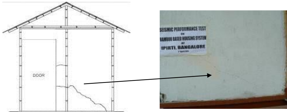
Figure 6(a): Front side crack pattern of Bamboo house
