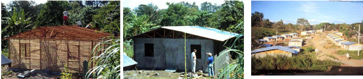
(a) Prefabricated panels (b) Plastered with cement mortar (c) A bahareque community
