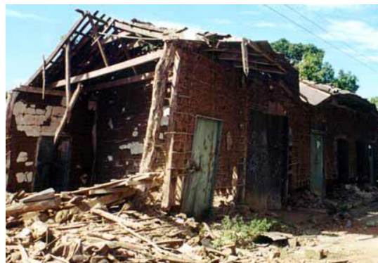
Plate 4 (b) Collapse of bahareque dwelling in San Agustín (13 January 2001 earthquake) (Lopez et. al., 2004[3])
