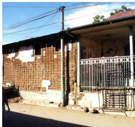
Plate 4 (a) Superficial damage to bahareque in Santiago de Maria 13 January 2001 earthquake (Lopez et. al., 2004[3])
